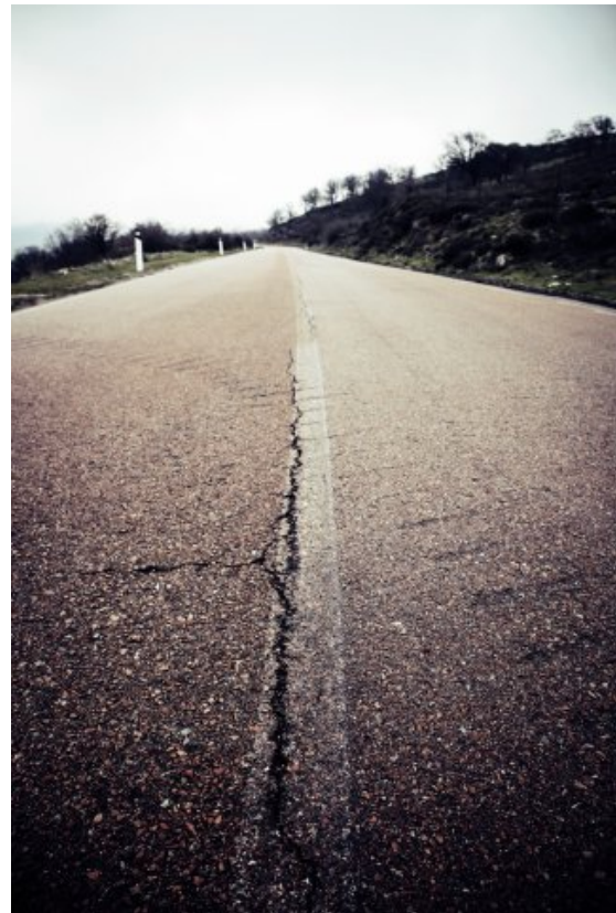
In Alaska, thawing permafrost has severely damaged airport runways, railroads, and pipelines. 16
